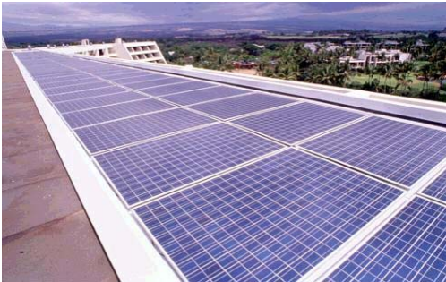
Figure 4 - Example of Interlocking Foam Insulating Panels Integrated with PV at Mauna Lani Bay Resort - Hawaii (Photo Courtesy of NREL and PowerLight Corporation)
