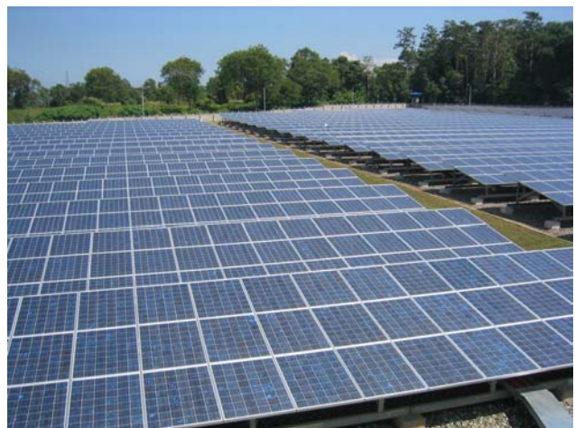
Fig. 1: CEPALCO 1MW PV system.
